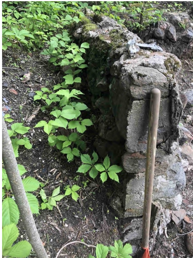
Photograph 20 Foundation 1. View of section of wall to the south of the feature entrance.
